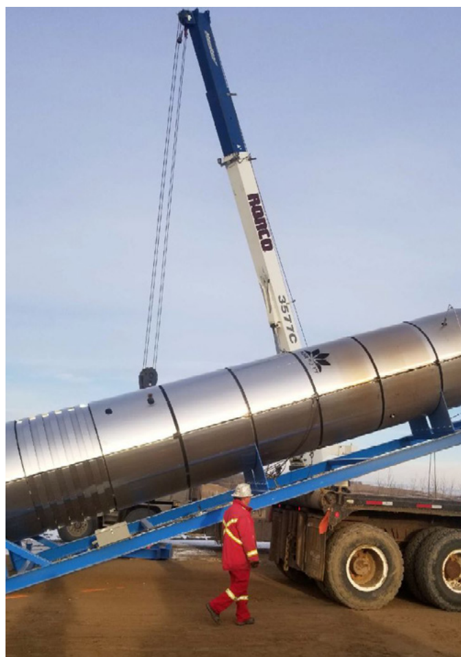
Testing a high-efficiency incinerator to combust methane.
