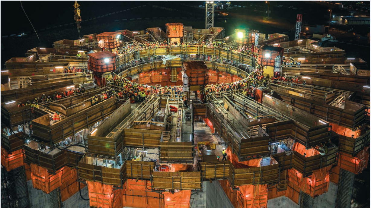
Workers mark the completion of the shaft in caisson slip at the West White Rose Project construction site in Argentina, NL.
